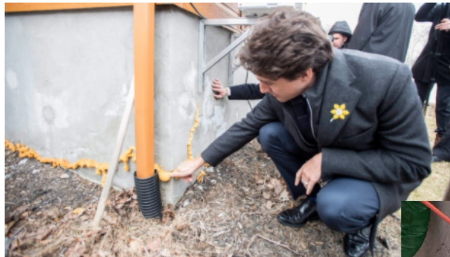
Prime Minister Justin Trudeau looks at the foundation of a house, in Trois-Rivieres, Que., on Wednesday, April 6, 2016. (THE CANADIAN PRESS/Paul Chiasson)
