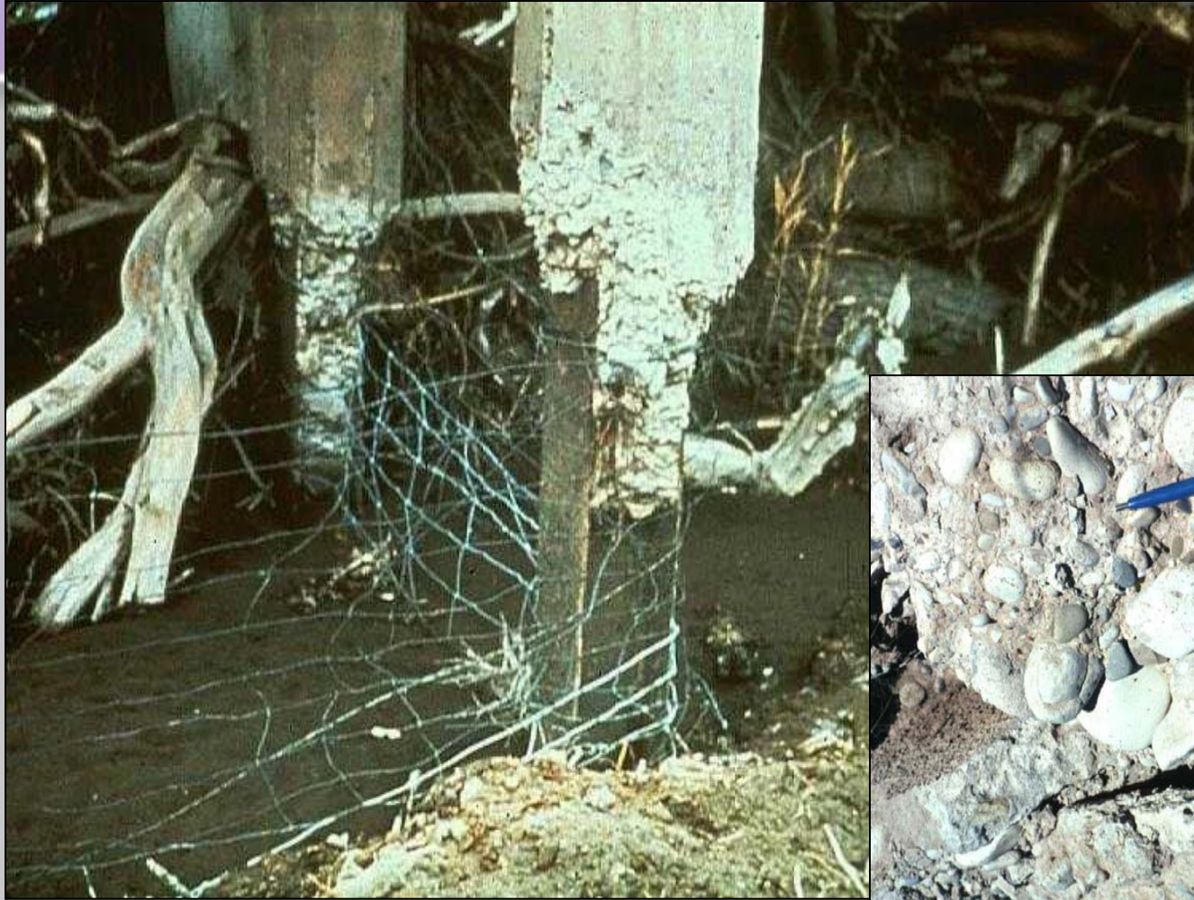
Bridge columns in North Dakota in sulfate soils
